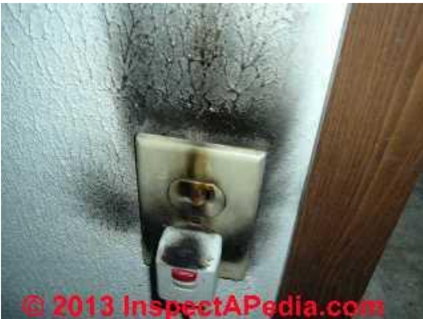
Our photo (above left) illustrates a burned-up electrical receptacle whose circuit was protected by a Zinsco circuit breaker that failed to trip and in fact had burned itself in the panel.
